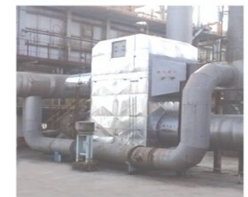
茂名石化240万吨/年渣油加氢装置 玻璃板式空气预热器 Glass Plate Heat Exchanger 2.4 million ton/year residue oil hydrotreating unit for Maoming Petrochemical
