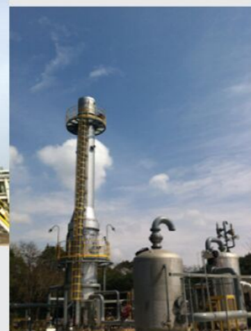
上海金山石化水务部有机废气处理装置 Organic waste gas processing unit Water Department of Shanghai Jinshan Petrochemical Plant
