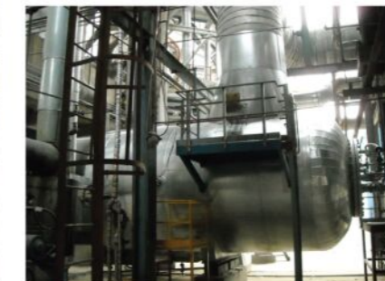
镇海炼化300万吨/年催化裂化装置 辅助燃烧室改造后现场图 3 million ton/year FCC equipment auxiliary combustion chamber site shoot after upgrade in Zhenhai refinery
